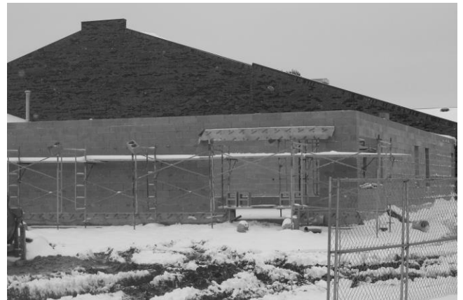
Teacher's Lounge area walls are up and waiting for the roof. (Adjacent to the library on the South side of the building)
