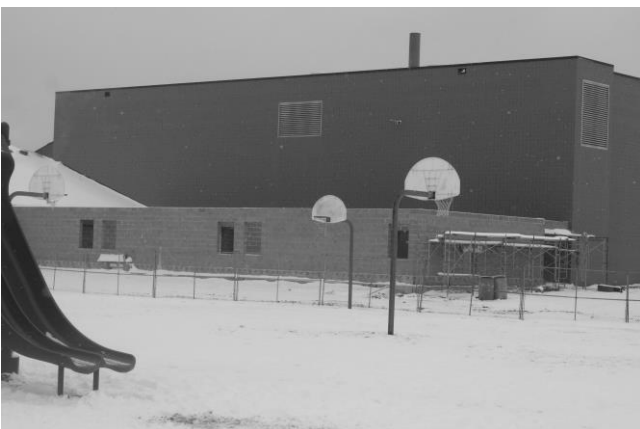
Three Junior High classroom walls are up, and waiting for the roof. (On the west wall of the Main Gym)
