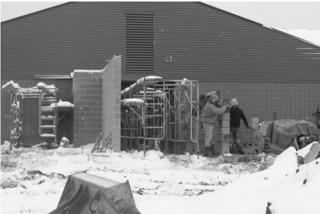
Beginning stages of the South classrooms (at the far SW corner of school)
